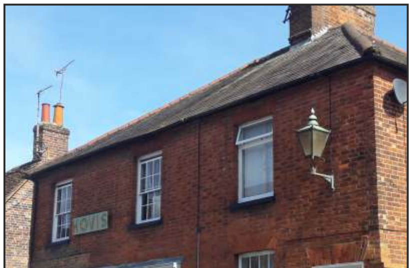
Replacement window on right side at first floor level is at odds with the original sash windows to the front elevation of 73 and 75 High Street
