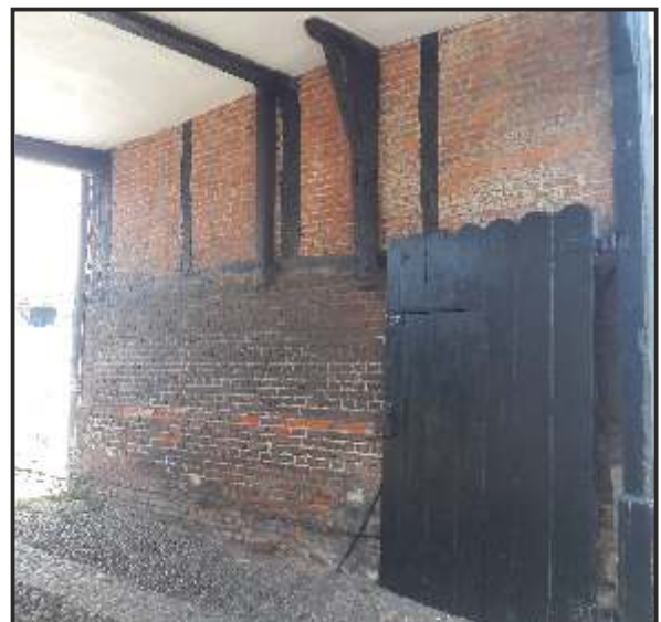
62 High Street, historic cobble surfacing within carriage arch containing timber frame and old red brick infill
