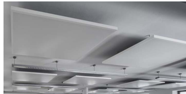
2. Ceiling canopy/panels – Cat B
