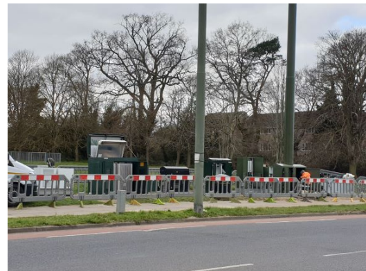
View of new Grovehill 5G Equipment Panels
