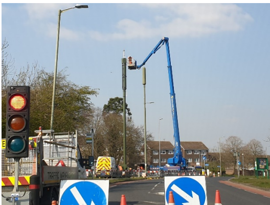
View of the new Grovehill 5G Mast Equipment Panels
