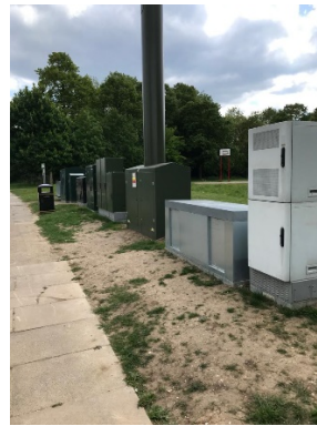
View of new Grovehill 5G Equipment Panels
