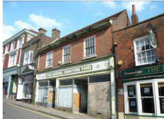
Figure 56: Nos. 21 and 21A a vulnerable buildings in poor condition requiring re-use
